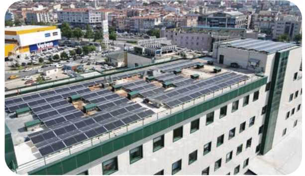
İstanbul Silivri Hospital / 100 kW
