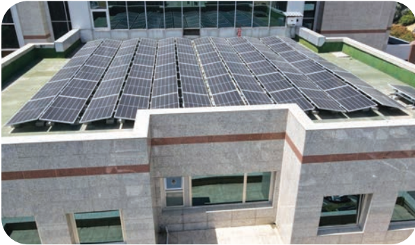
İstanbul Başakşehir Hospital / 30 kW
